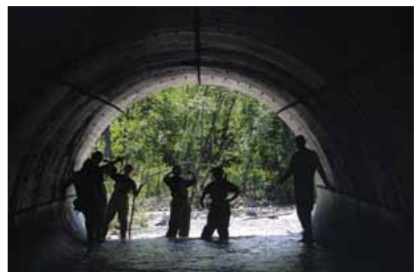
Although this culvert seems huge, we were able to see adverse effects on the hydrology of the creek which in time could hinder passage of fish.
